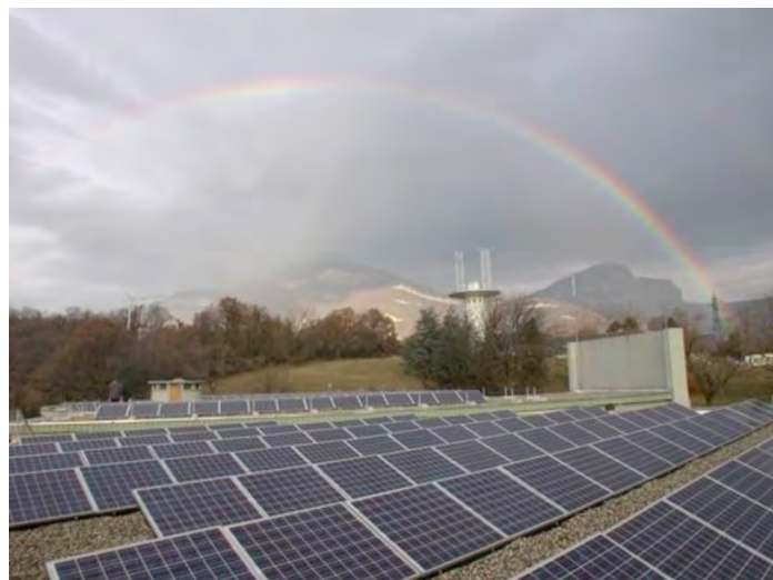
Photovoltaics panels on a roof terrace, Chambéry, France. (HESPUL)
